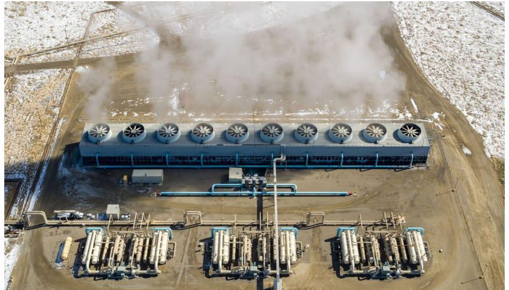
Fervo Energy 3.5 MW EGS Pilot in Nevada
