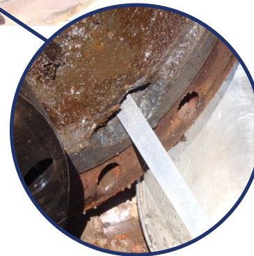
SRB pitting corrosion of pipeline flange end
