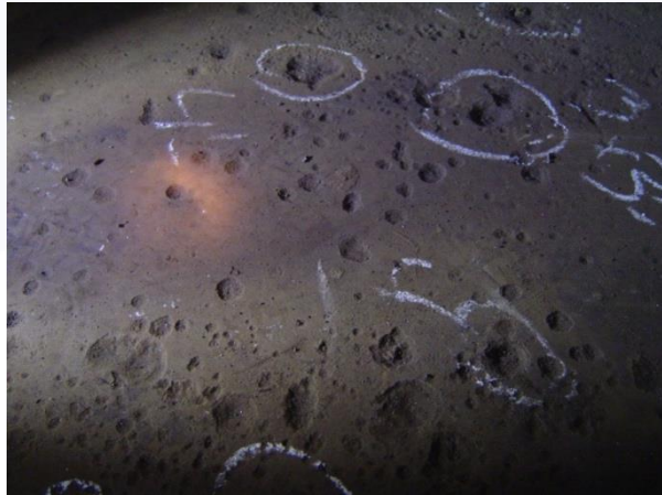
SRB pitting corrosion of tank floor
