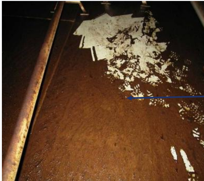
Microbial biofilm in jet fuel storage tank
